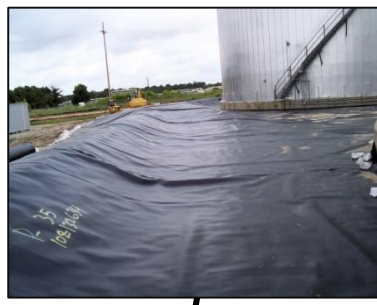
Tank Berm Containment
